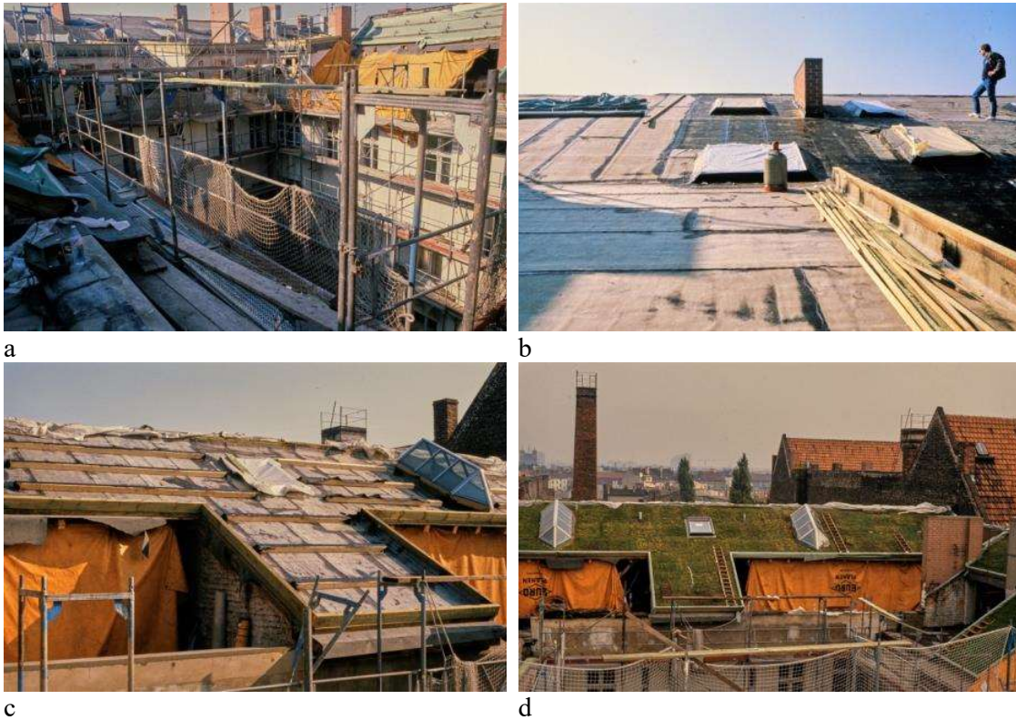
Figure 2a–d. Details of the green roof installation in September 1985. Upper row: Scaffolding and lifting the older roof to construct the roof level apartments. Lower row: Installation of the thrust-thresholds and the PVC layer. Lower right: With the final turf mat layer.
